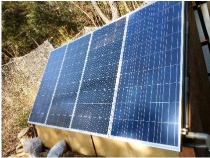
Solar battery panels for the equipment installed on-site
