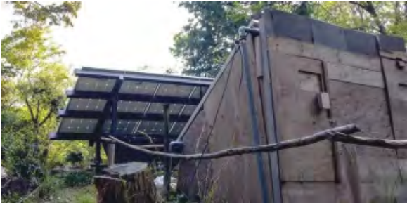
Solar battery panels powering the on-site equipment
