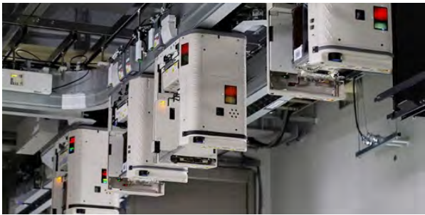
Transport equipment inside the clean room
