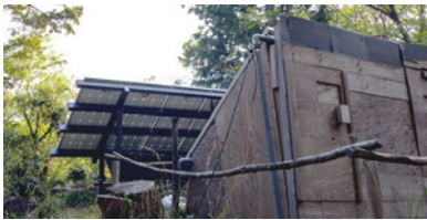
Solar battery panels powering the on-site equipment
